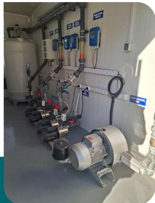
Figure 5. Interior of the ITU WWTP, highlighting its compact design. Source: Ibn Tofail University
