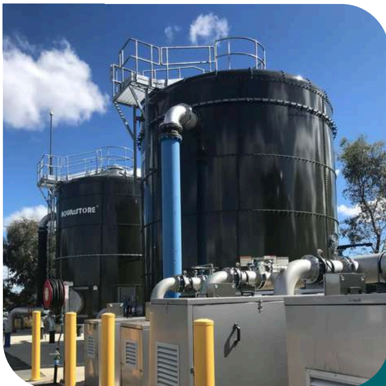
Figure 3. Recycled water storage tanks. Source: Australian Water Association (2023).
