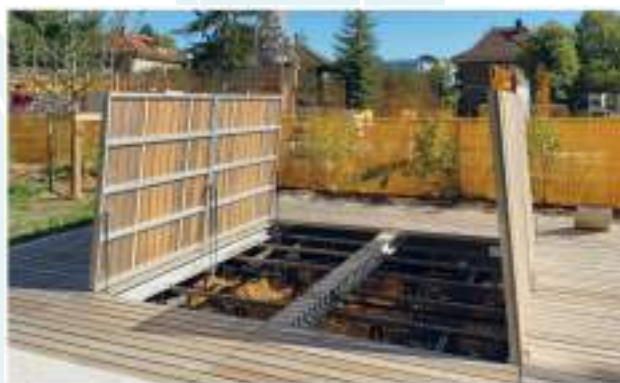
Composting system situated under a terrace. Equilibre housing complex Soubeyran, Geneva. Source: Cooperative Equilibre
