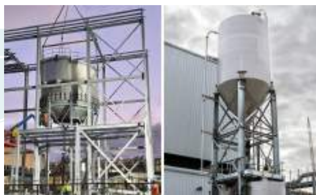
Ringsend WWTP Phosphorous reactor (left) and magnesium oxide storage silo (right). Source: Water Projects | Murphy Ireland
