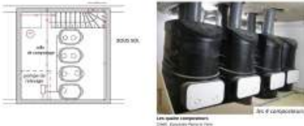
Four composters at the basement of the St Germé school, France. Source: OCAPI | Pierre et Terre
